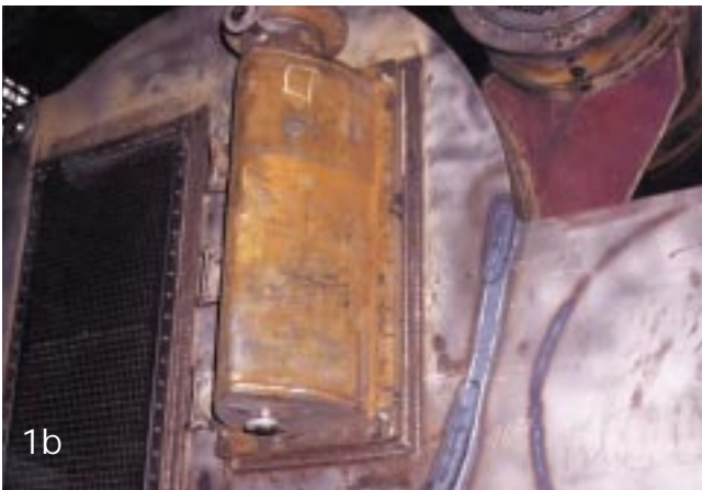
Figure 1: Heat exchanger for hydro thermal water.
